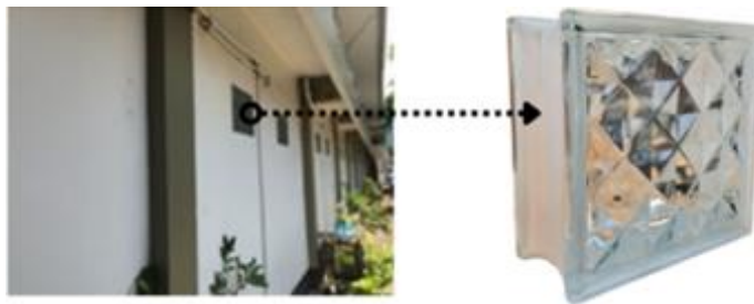
Gambar 1. Ventilasi glass box
